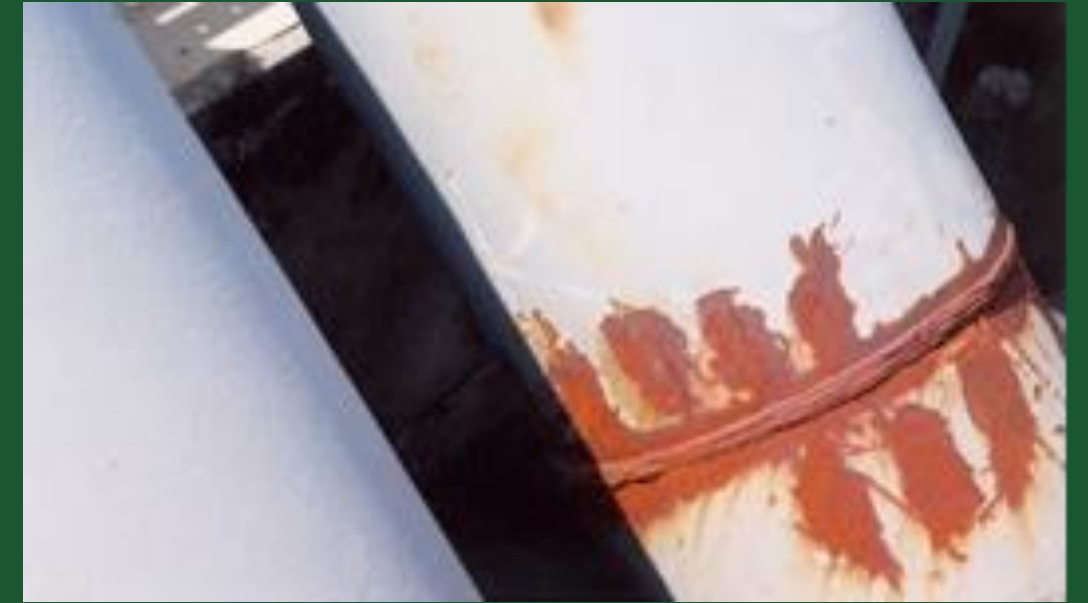
Figure 1: Heavy rusting around welds were cleaned by power tools to tightly bound rust
